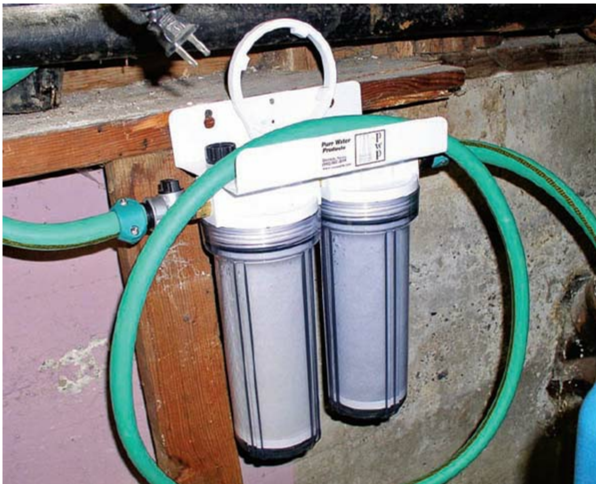
This carbon filtering unit removes chloramine among other things
